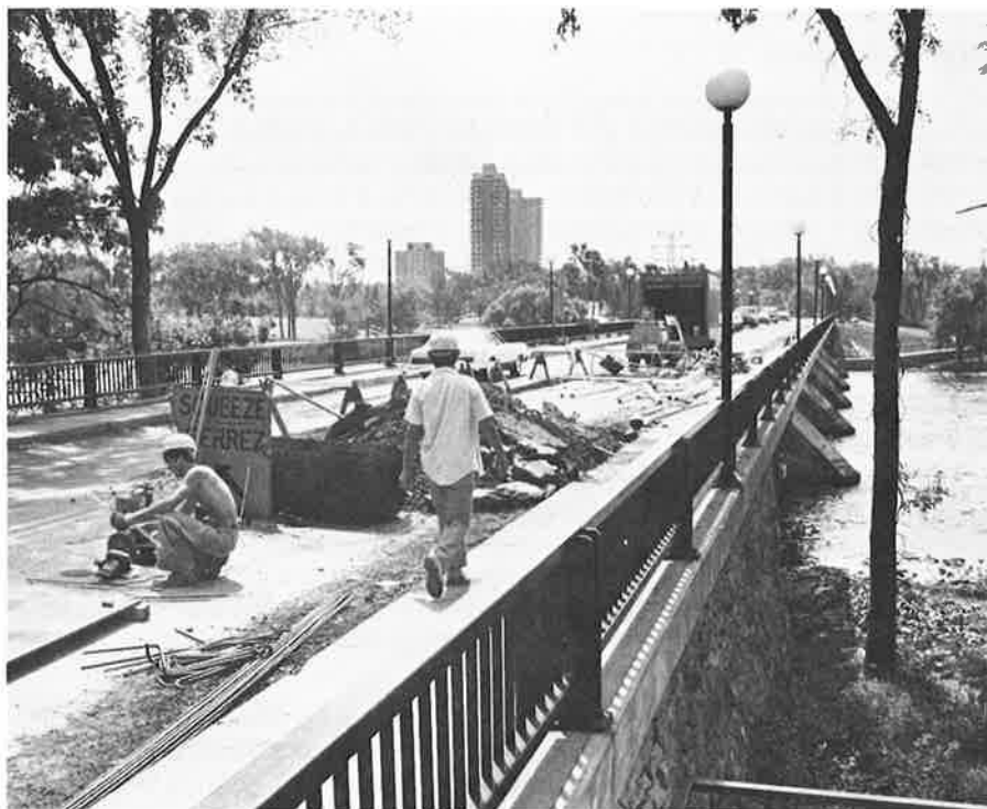
The Champlain Bridge, maintained by the NCC, is more than 50 years old and needs repair.
