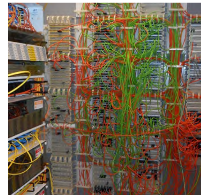
FIGURE 64. SERVER ROOM, STRUCTURED CABLING SYSTEM Source : Stantec
